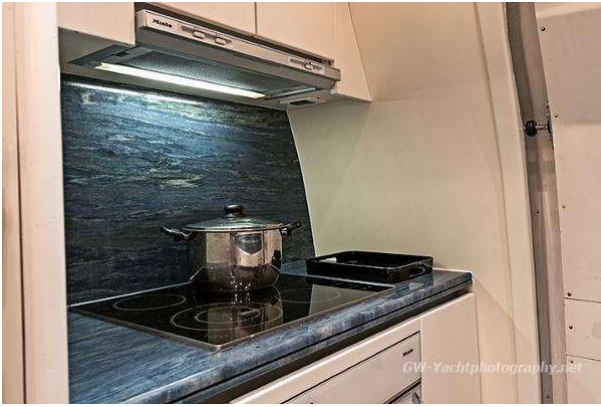
Galley Cooking area
